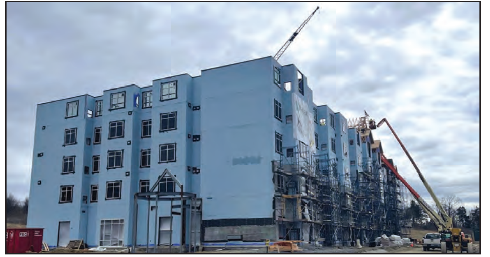
Construction work progresses at the Bellefield at Historic Hyde Park site, across Route 9 from the Culinary Institute of America in Hyde Park. Courtesy photo
